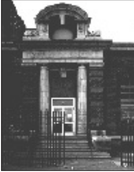
Entry at Bushwick Branch in need of restoration
