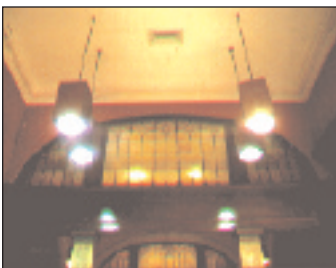
Inappropriate pendant lights at Park Slope Branch
